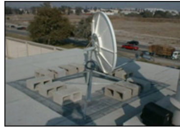
DPAS system built to offer 60 USFS users network connectivity
